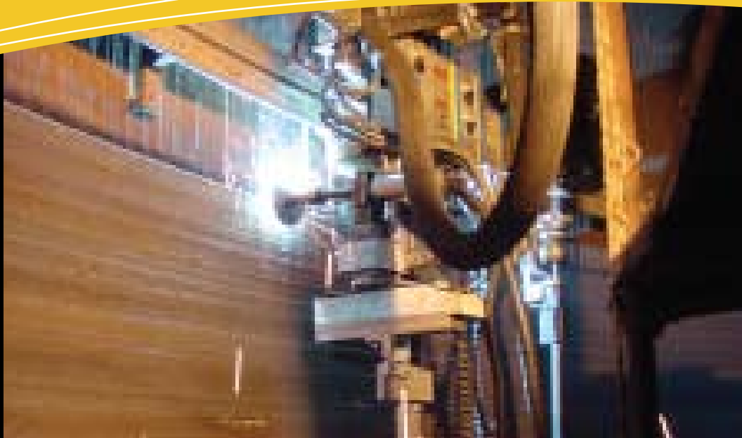
Figure 1. Unifuse® overlay welding machine performing overlay welding for a vessel. The bottom half of the photograph shows a newly applied overlay on the vessel shell.
